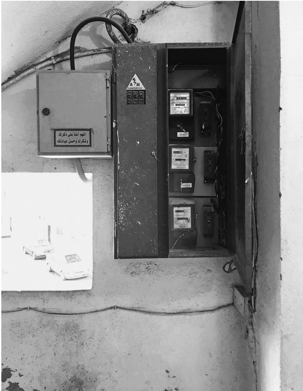
Figure 4. Image of electricity meter boxes installed by the Jordanian Electric Power Company. Photograph by the author, 2019.
